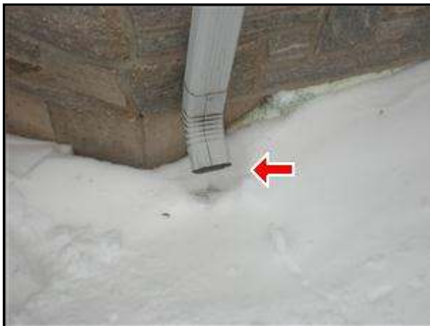
2.6 Picture 1 Missing gutter Extension
