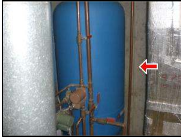
7.5 Picture 1 water storage tank
