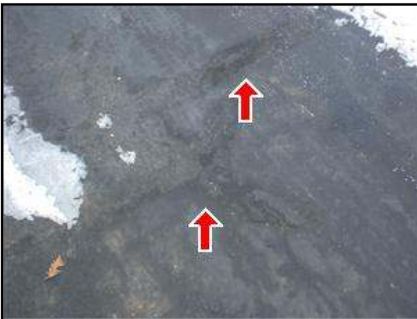
1.13 Picture 1 Driveway cracking
