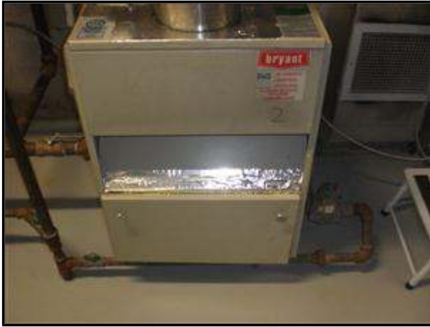
5.0 Picture 1 Heating System
