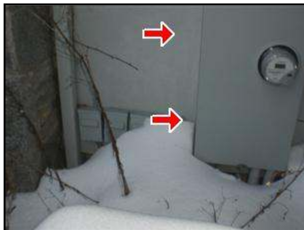
1.17 Picture 1 Electrical Service Entry
