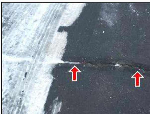
1.13 Picture 3 Driveway Cracking
