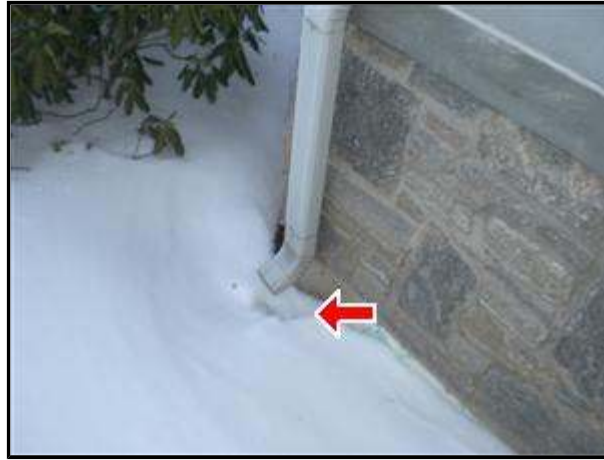
2.6 Picture 3 Missing extension
