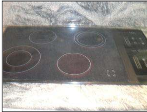
8.9 Picture 1 Stove top not functioning
