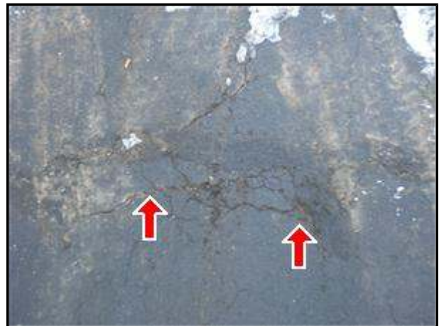
1.13 Picture 2 More Driveway cracking
