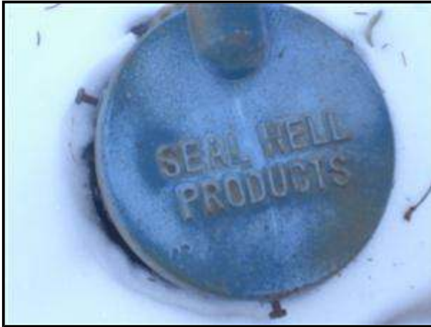
7.0 Picture 1 well head
