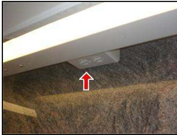
Kitchen outlet not GFI
