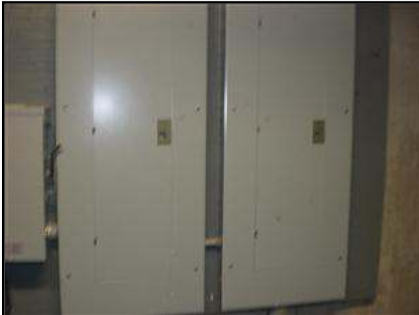
6.1 Picture 3 Electrical Boxes
