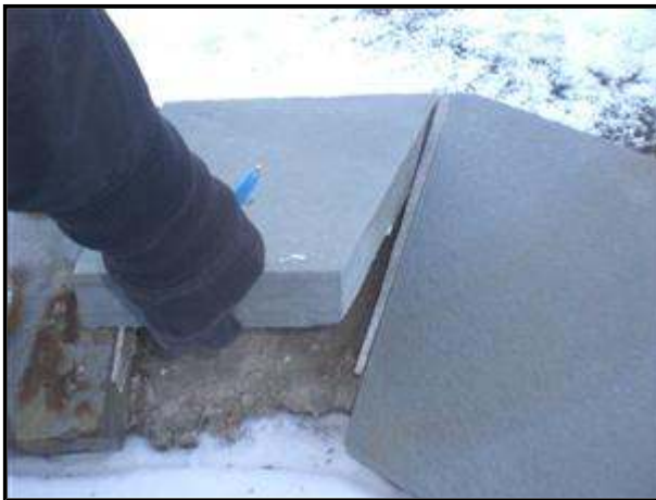
1.5 Picture 1 Front retaining wall cap loose
