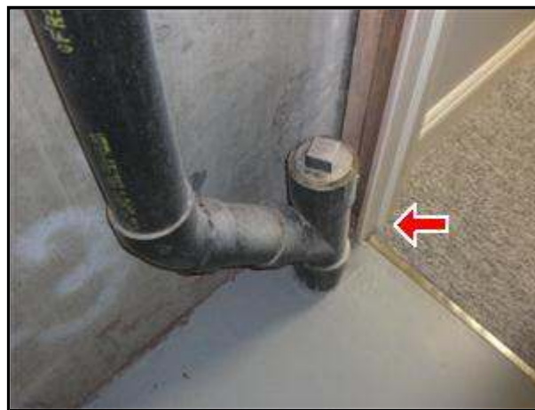
7.4 Picture 1 waste pipes
