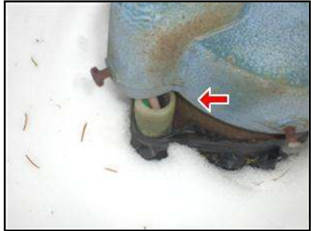
7.0 Picture 2 well head wiring open to elements
