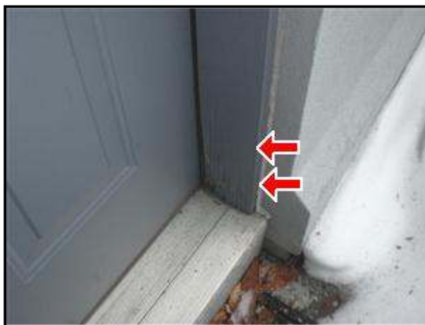
1.15 Picture 1 Rear door framing rotting
