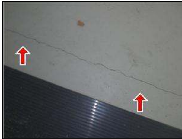
3.1 Picture 1 Garage Floor
