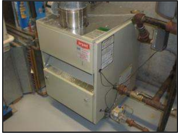
5.0 Picture 2 Heating System
